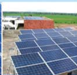
100 kW Solar Rooftop project at VVIT, Guntur, Andhra Pradesh
