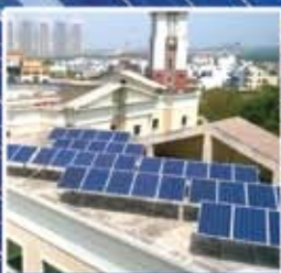
77 kW Solar Rooftop project at Suncity School, Gurgaon, Haryana
