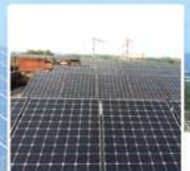
192 kW Solar Rooftop project at IIT Kanpur, Uttar Pradesh
