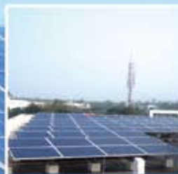
200 kW Solar Rooftop project at Vishnu, Bhimavaram, Andhra Pradesh
